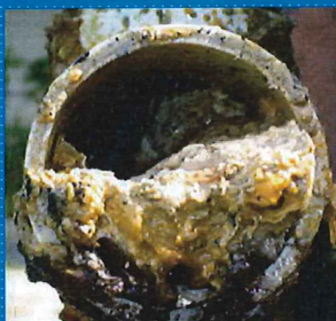
Grease that was poured down kitchen drains & from poorly maintained grease traps
