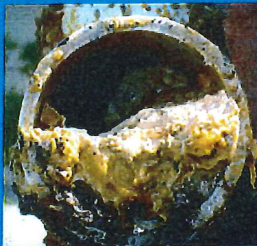
Grease that was poured down kitchen drains & from poorly maintained grease traps
